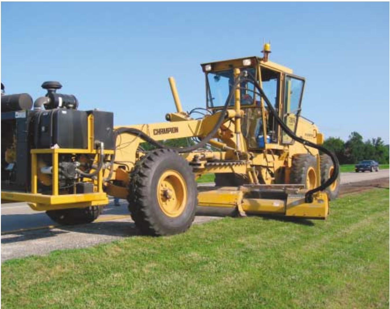
Mounted on a MODOT motor grader, the RotoGrader grinds and pulverizes the old shoulder material on Route 61. Power for the attachment comes from the front-mounted diesel engine.
