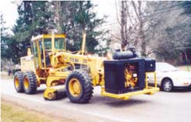
A passing car demonstrates one of the benefits of the RotoGrader: it can mill pavement in one lane without obstructing traffic in the other.
