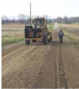
The powerful rotary action of the cutter drum provides uniform penetration and excellent gradation of the surface material.
